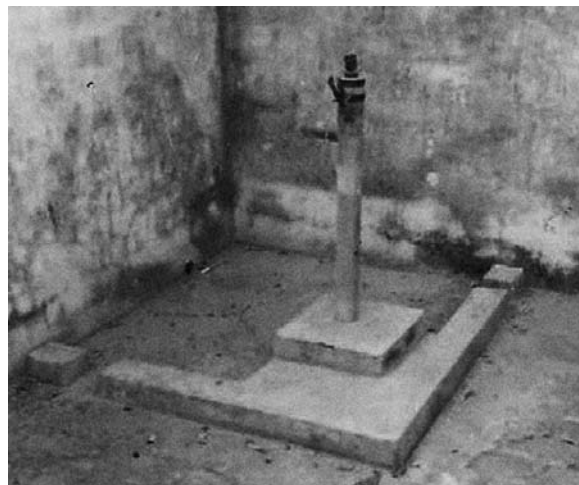
Non-functioning hand pump at health center, Uttar Pradesh
