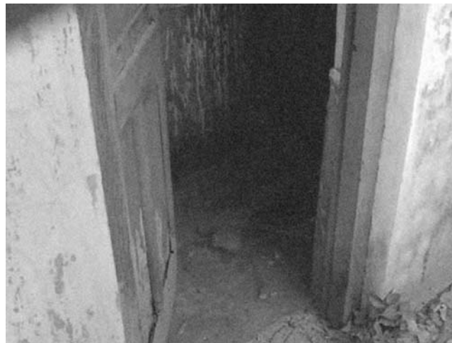
Toilet in primary health center, Uttar Pradesh
